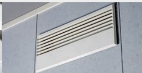
Linear slot and wall diffusers
